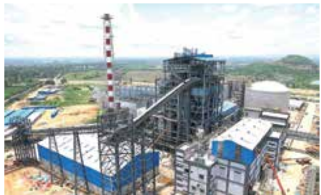
▲ Aerial view of the Captive Power Plant at Gopalpur.
