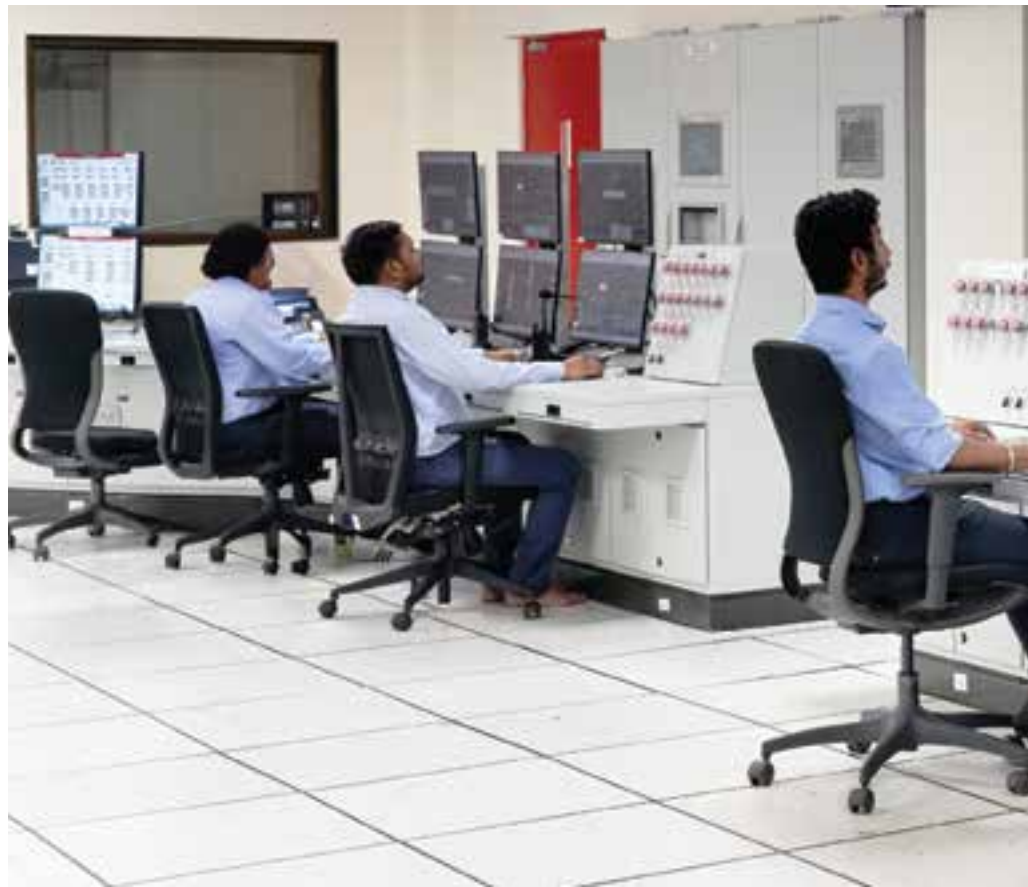
▲ State-of-the-art Main Control Room of the Ammonia Plant at PCL Talaja.
